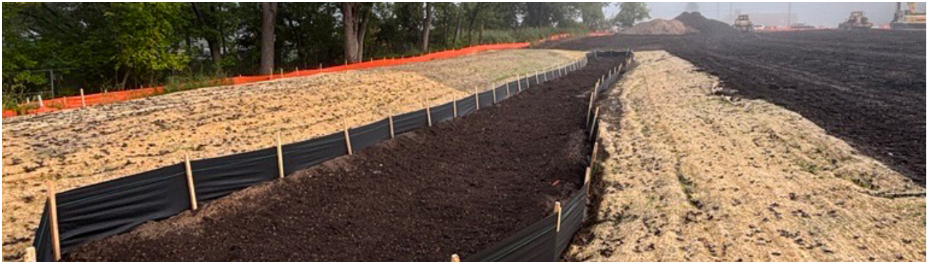
Construction site erosion control practices around an infiltration basin (black fencing) and site perimeter (orange fencing)
