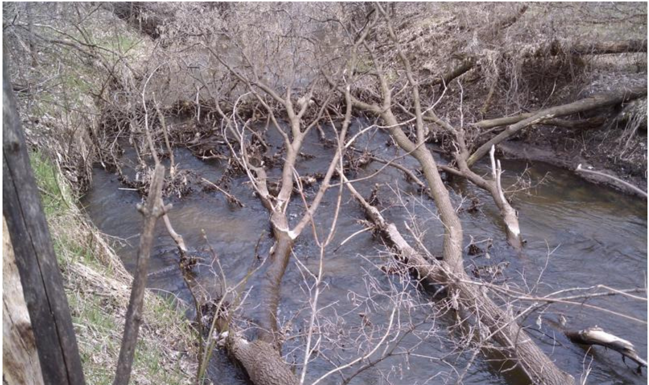
Sand Creek Obstruction at Xeon Street 2011
