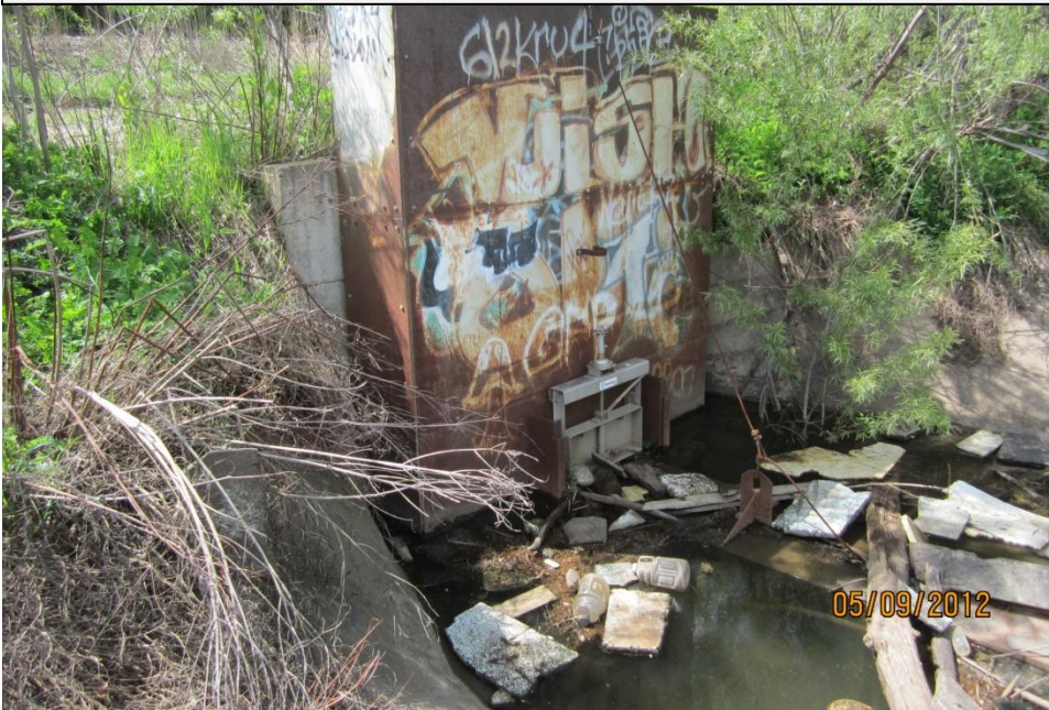
Structure on upstream end of Rail Road. Accumulation of debris.
