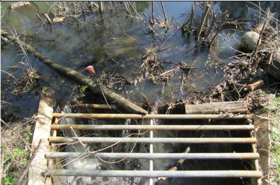
Obstructed trash rack on upstream end of 96 th Lane NE. Temporarily relieved 5-18-2012.
