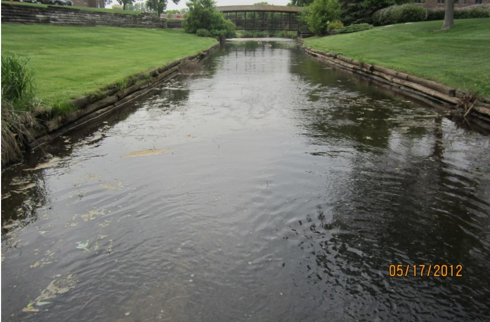
Pond created by wood weir upstream of Coon Rapids Blvd. Accumulation of animal feces (primarily goose).
