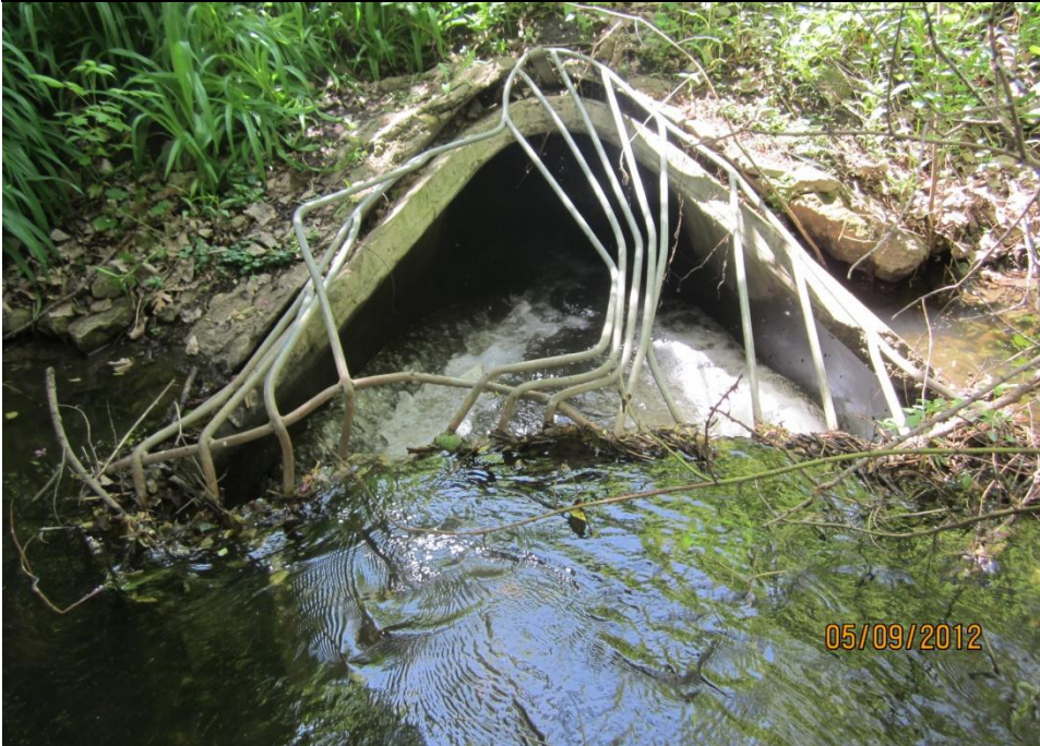
Obstructed trash rack on upstream end of Norway Street. Temporarily relieved 5-9-2012.
