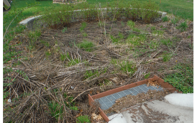
The matted brown vegetation in this rain garden needs to be removed. The Rain Guardian pre-treatment device needs to be cleared of leaves and its top grate should be removed so the inner chamber can be shoveled out.
