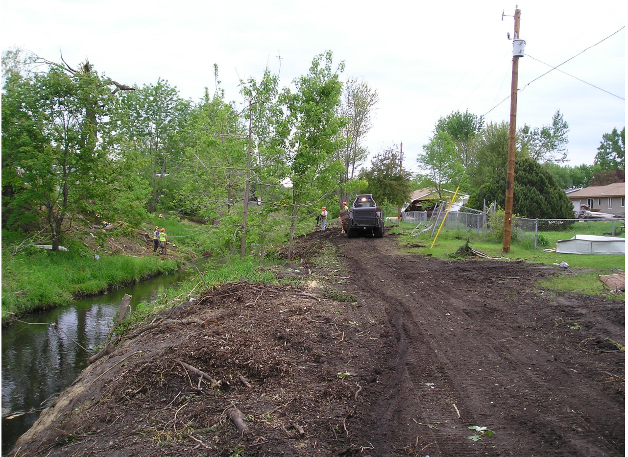
Tornado clean up on Sand Creek (Ditch 41) Blaine & Coon Rapids May 2008
